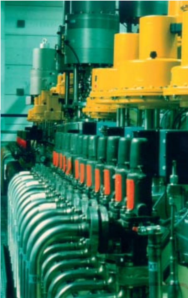
A complicated system of valves distributes liquid helium to the superconducting magnets of the HERA ring.
