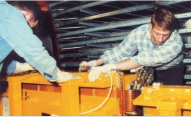
Setting up the heavy magnets is a high-precision job. All the parts have to fit together with a tolerance of a few tenths of a millimeter.
